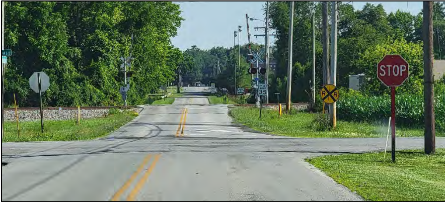
Photo 1: Looking northward on Beeler Rd. at Breese Rd. where the NE corner has tight turning radius for school bus movements
